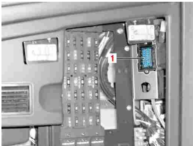
Driver's area interior switch panel
